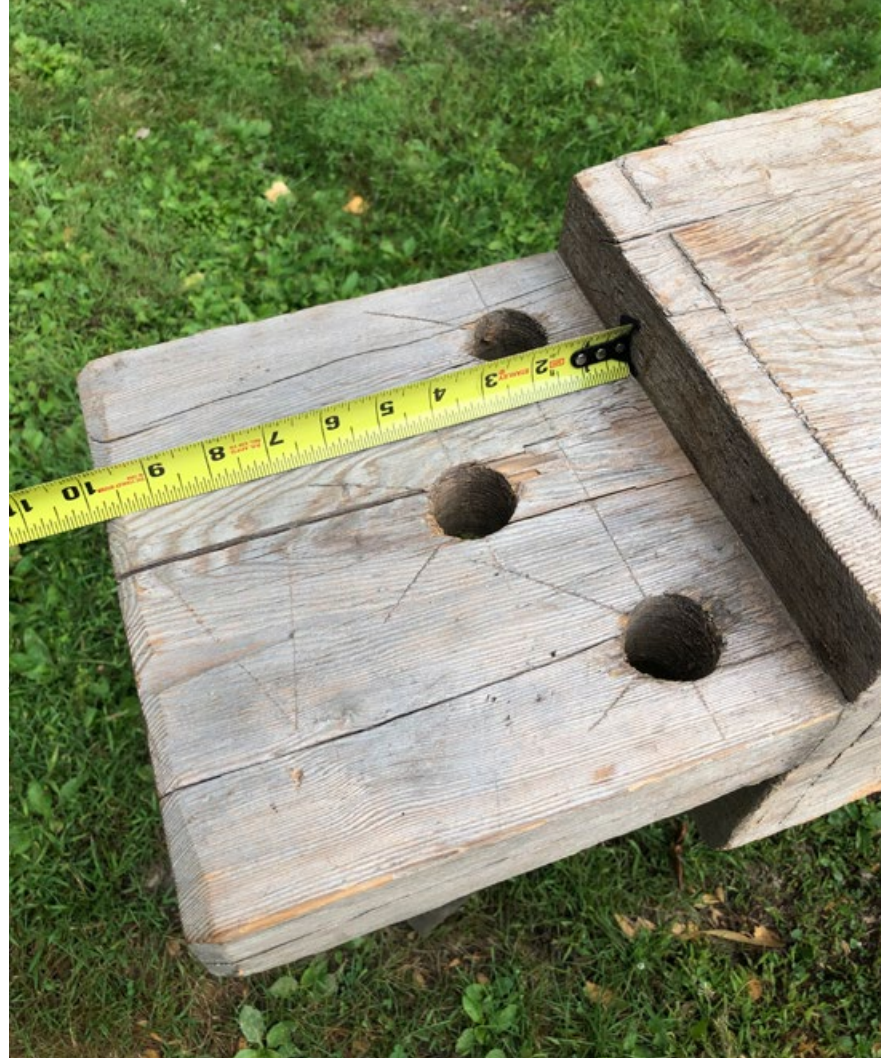
4 This early-19th-century 10x12 tie beam end has a 2\frac{1}{2} -in.-thick tenon, 2 in. off the face, with three 1\frac{1}{2} -in.-diameter peg holes. The 2- and 4-in. spacing off the shoulder is clearly seen. The drawbore offset here measures \frac{3}{32} in.
