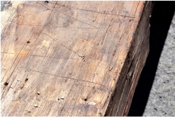
3 This old timber shows the square-ruled layout for two peg holes on a mortise that was never cut (a layout mistake). Looking closely, the line for the housing (near right edge) and the parallel line for the peg holes at the point of the carets can be seen.
