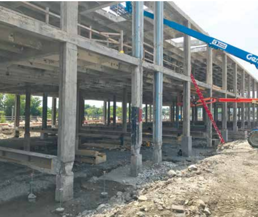
Figure 2. The crumbling concrete carcass before the transformation.
