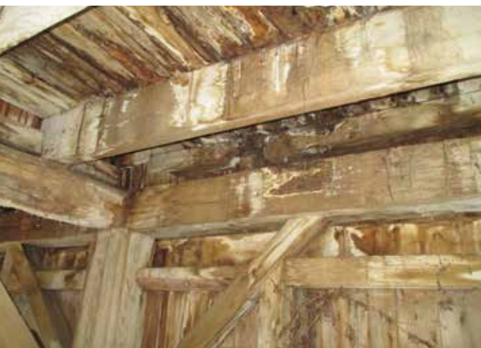
Wet discolored timber is evidence of decay.
