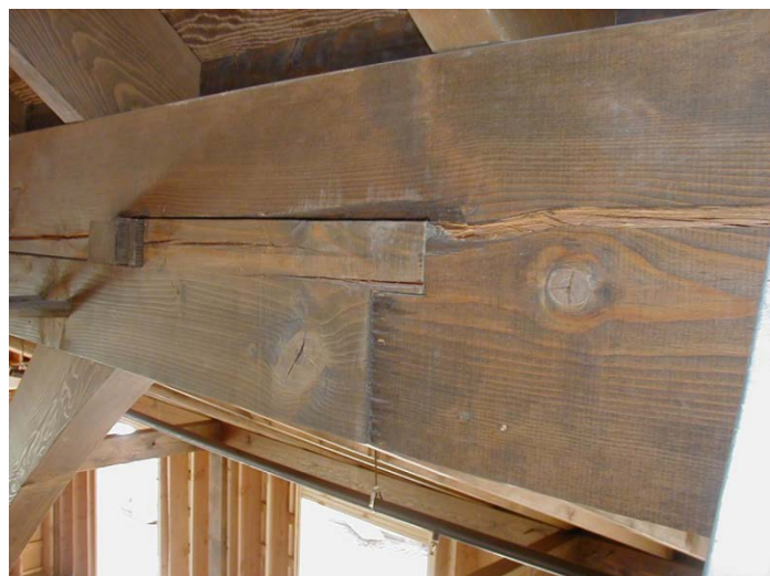
Figure 3 Failed scarf joint
