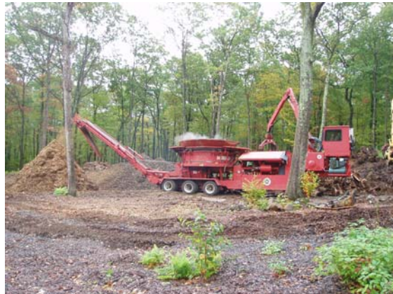
Figure 10 Wood construction waste is converted to landscape mulch in a tub grinder. Photo by DeStefano & Chamberlain
