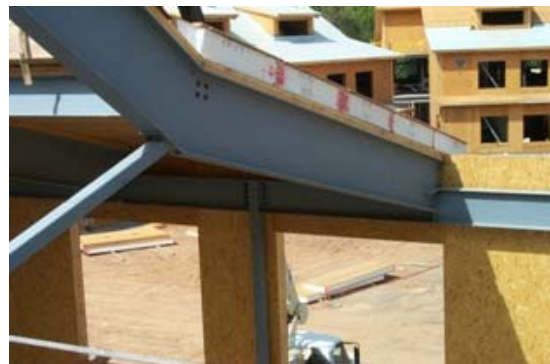
Figure 7. SIP roof and wall cladding over structural steel on a school in Cherokee, NC. Photo by Panelwrights.
