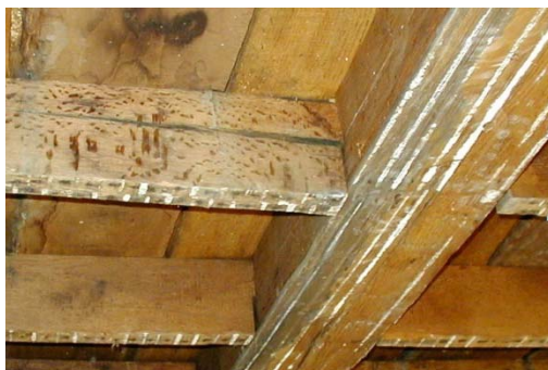
Figure 2 - Failed Butt-Cog Joint
