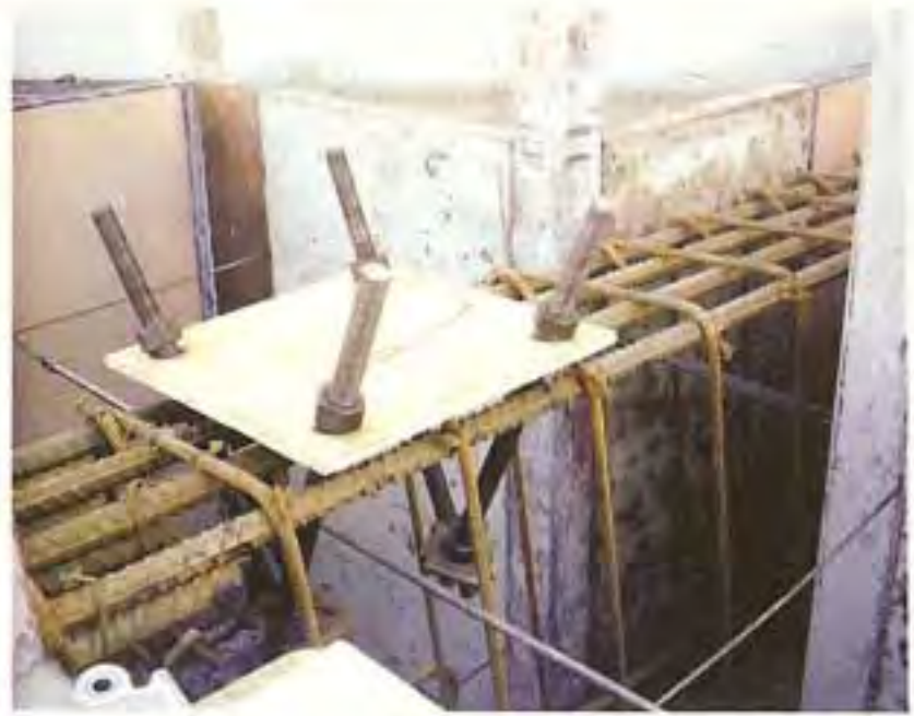
Errors can be easily corrected when SERs manage special inspections. Inspectors on this jobsite reported that the anchor bolts were found to be in the correct location, but not perfectly plumb.
