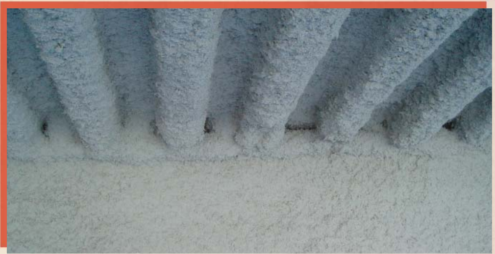
Flutes of metal deck have not been completely filled over beam
